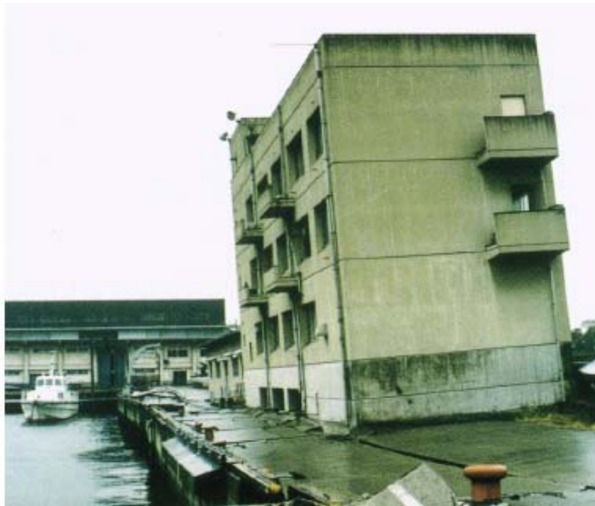
Figure 1: Failure of a pile-supported building during 1995 Kobe earthquake
