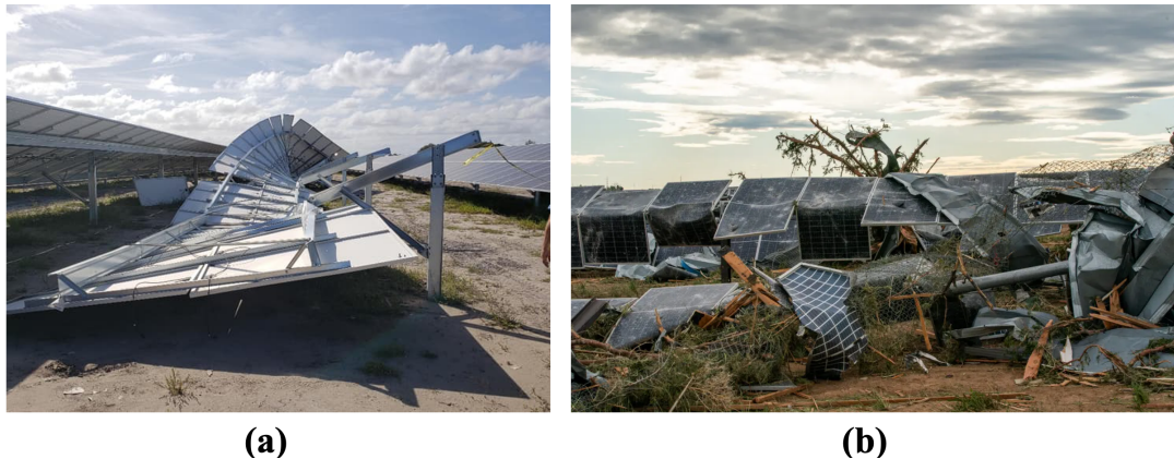
Figure 1. Example of damage to solar panels due to high winds. (a) Overturning failure; (b) complete damage.
