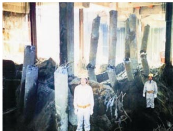
Figure 3. Excavated piles of a building twenty years after the 1964 Niigata earthquake. The superstructure is three-storey RC building. The piles are precast RC piles 10 m long and 300 mm in diameter. (Photo courtesy: T. Tazon.)
